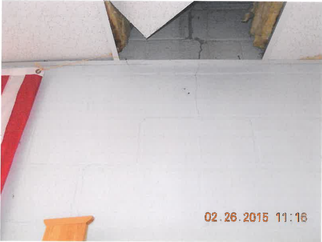
Old crack noted by mortar repair
